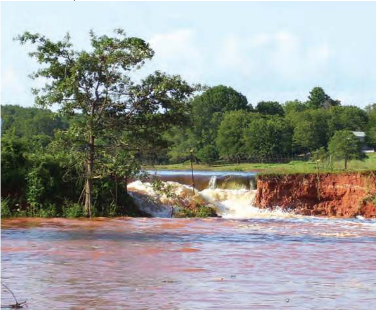
FIGURE 3.1 EMBANKMENT DAM FAILURE IN CLEVELAND COUNTY, OK
