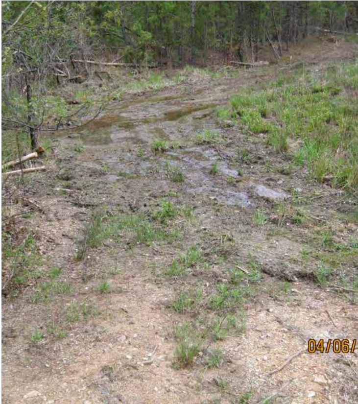
FIGURE 5.5. AREA OF SEEPAGE NEAR TOE OF DAM.
