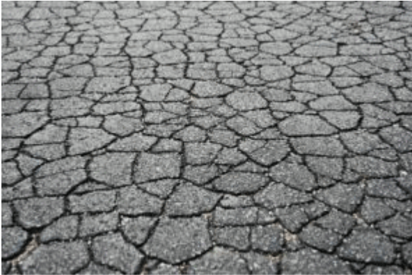
Example of alligator cracking (photo is NOT from HSV and is for illustrative purposes, only)
