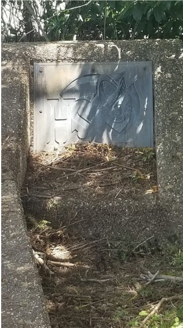
Uncleaned Brass Plate at Bridge at Danville Gate/Baleric
